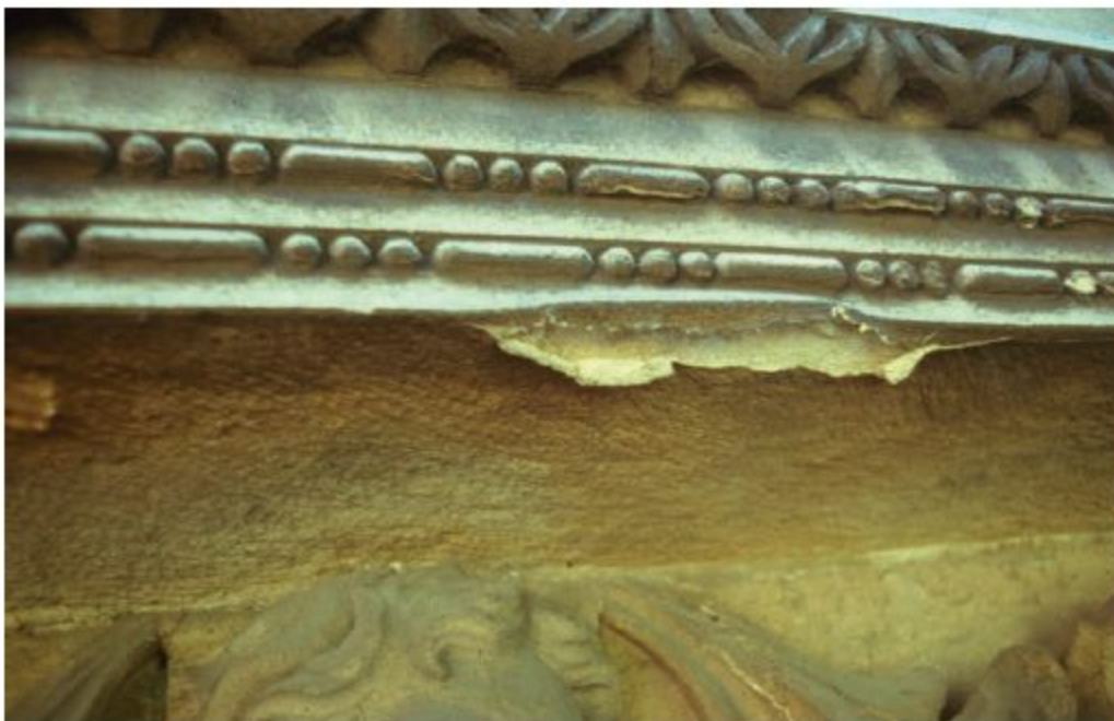
Figure 2.4 Damage caused by calcium sulphate crystals.
