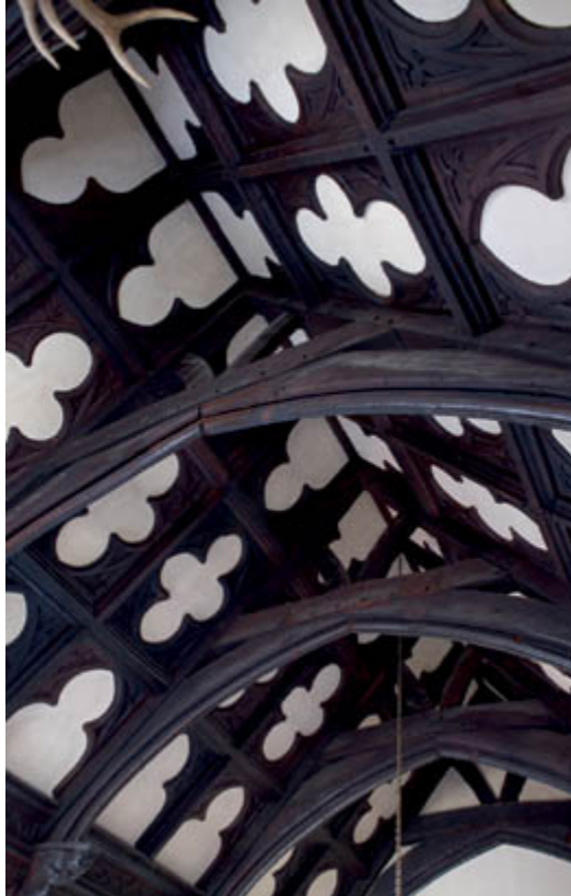
The early fifteenth-century roof timbers of the Great Hall are ornate and intended to be seen and admired. Particularly striking are the arch-braced collars and cusped wind braces.
