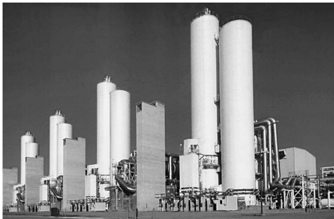
Fig. 1.3 Air separation unit at Cantarell, Mexico (2000).
