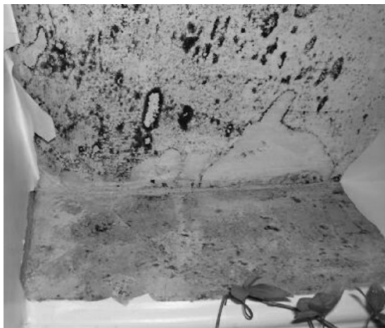
Fig. 1.6 Part of a bathroom ceiling where the paint has flaked away, revealing extensive growth and sporulation of sooty moulds.
