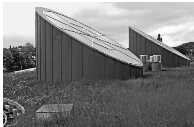
FIGURE 2-3 This living green roof has a 6-inch soil profile and is covered with a matrix of grasses. (Photo: Kai-Henrick Barth)
