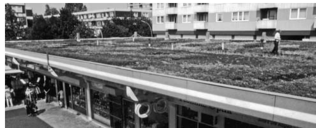
FIGURE 1-11b This living green roof is over a parking structure that is part of a shopping center in the central business district of Nürtingen, Germany. The living green roof is primarily used for stormwater management, but it also adds a visual amenity for the residents and office workers in the adjacent building. Additionally, it offers limited access for shoppers, residents, and workers wishing to walk through the living green roof garden. (Photo: re-natur, 24601 Ruhwinkel, Germany)
