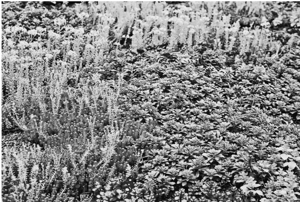
FIGURE 1-10 Although a number of species of the genus Sedum may be utilized, a balanced matrix of genera should be included in the plant palette of a living green roof.
