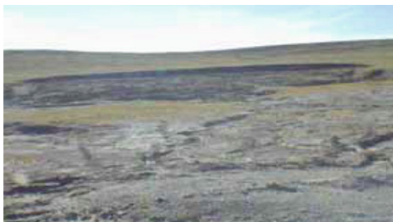
Fig. 2 Thaw slumping near milepost K3035 of QTH
