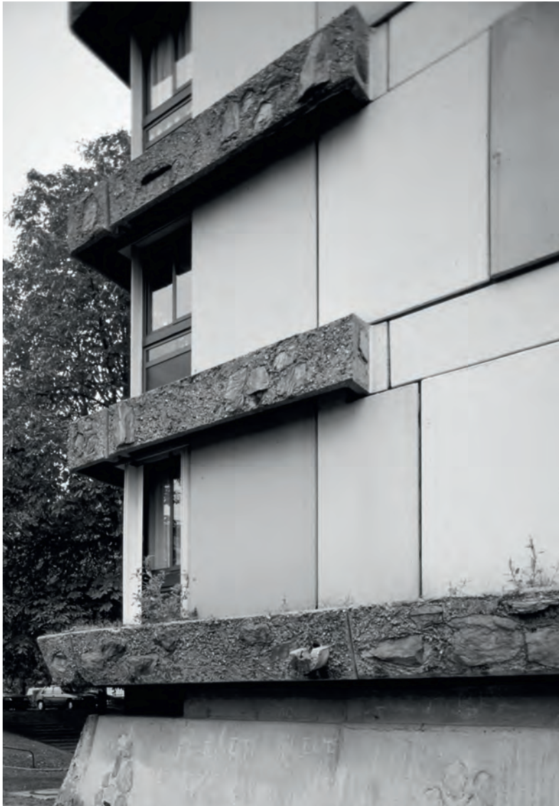
Les Bleuets housing estate in Créteil, Paris (1959), designed by Paul Bossard and featured by Adrian Forty in Concrete and Culture (2012).
