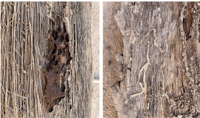
Fig. 23.12 Particular termites attack along the core of the beam, well visible through the condition inside the canals and by typical tunnels around the deeply damaged part. The particular termites' typical tunnels on a date palm beam are visible on the right (author's photos)
