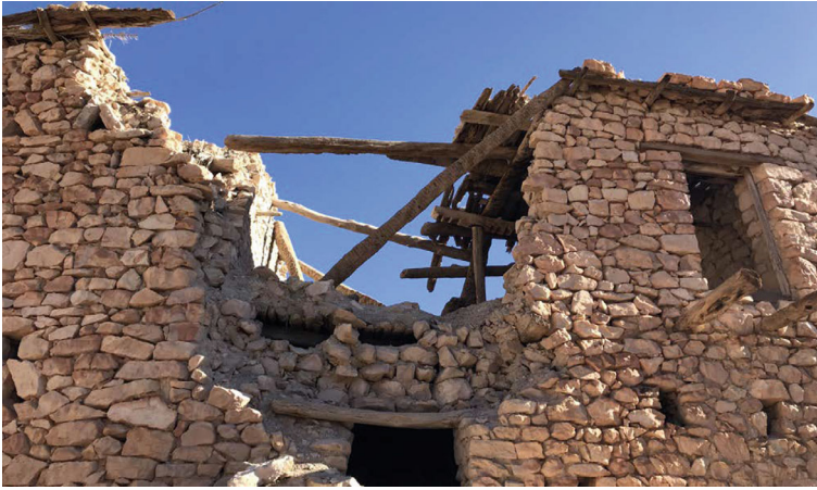
Fig. 23.13 Even in severe conditions, wooden elements seem more resilient than stone elements in a lack of maintenance intervention (author's photo)
