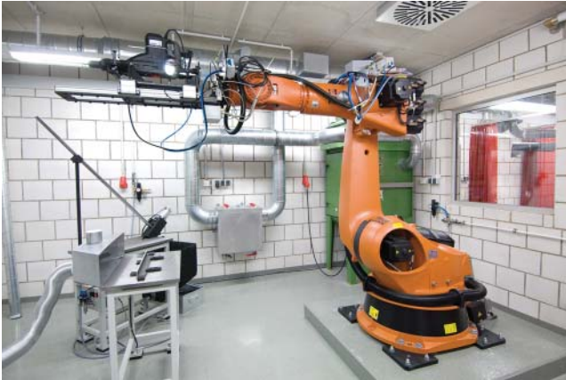
Figure 1.6 Industrial robot fastened with anchors (photo: Künzlen).
