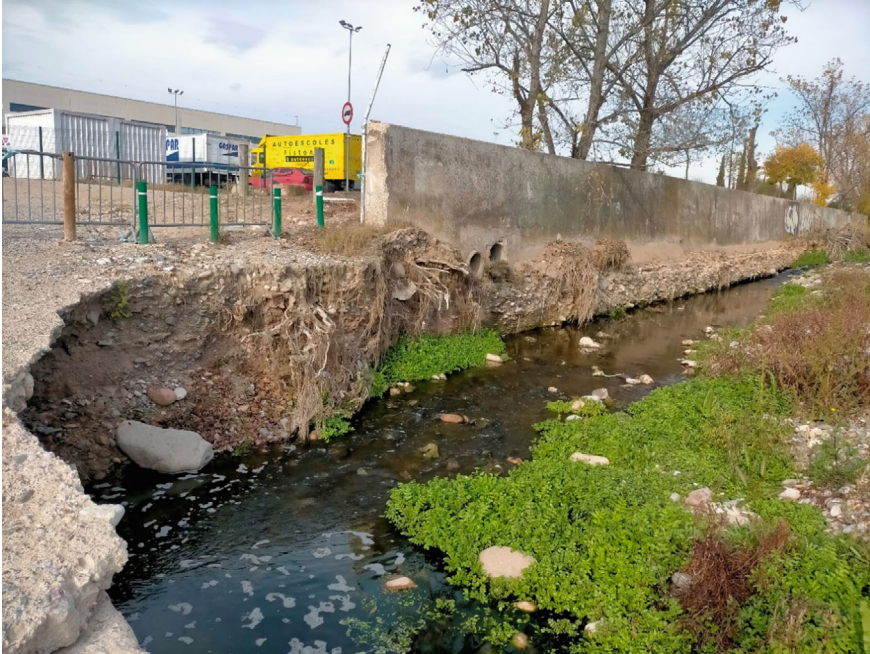
Fig. 1.1 Undercutting of flood protection walls on the river Congost in Granollers (Barcelona, Spain). Source Joaquim Farguell (October) 2022
