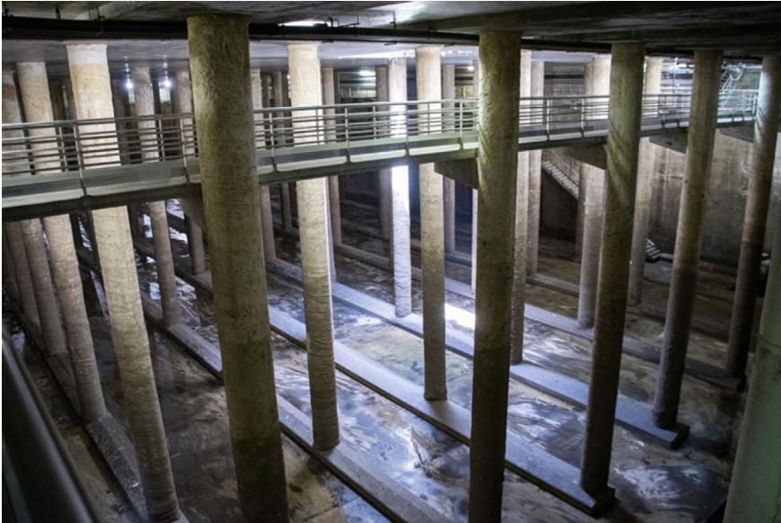
Fig. 1.6 Stormwater tank (SuDS) in Barcelona for the storage of urban surface runoff from rainfall events. Source Barcelona City Council. Stormwater tank plan (Universal access)
