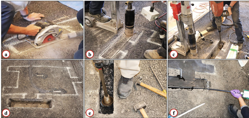
Fig. 9 Capacitor unit installation process; a sawing, b coring; c compacting; d cleaning; e pouring some asphalt and compacting; f fixing capacitor box with resin/epoxy
