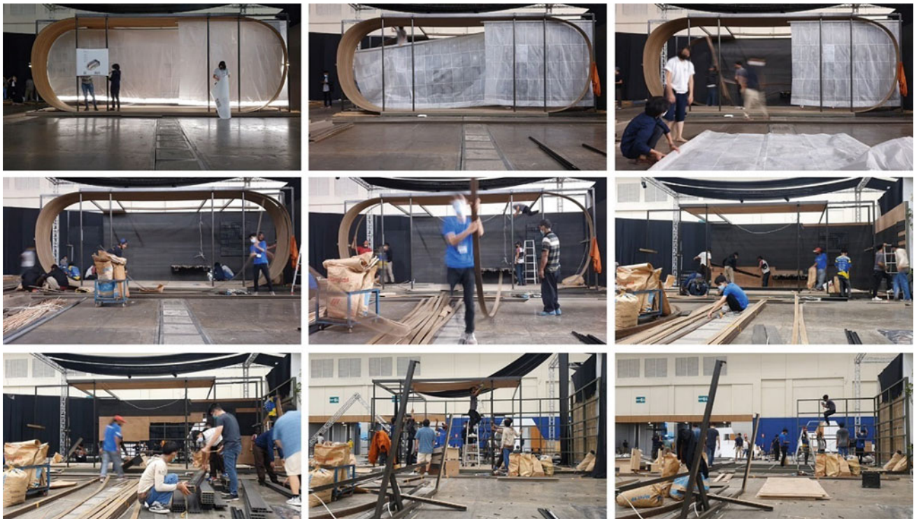
Fig. 10 In the dismantling process, all materials were sent back to their manufacturers. Source monokroma architect
