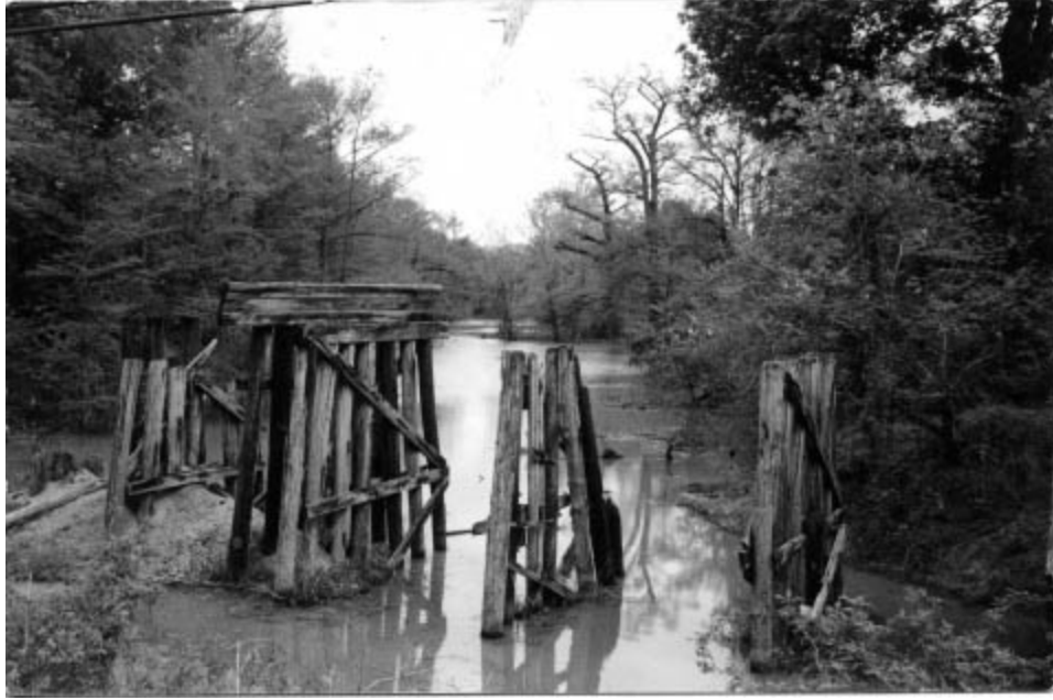
The ruins of a bridge, Mississippi Delta
