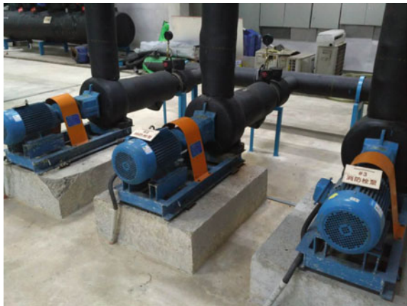
(b) A building with power equipment
