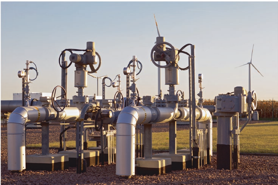
Fig. 1.4 ONTRAS compressor station Bobbau (Saxony-Anhalt). (Source: Ontrans – Photo: Peter Eichler)
