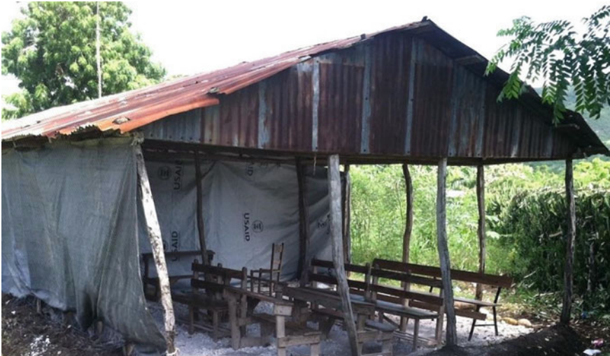
Fig. 2.1 'Secondary school classes are held in this space. Classrooms are separated by tarpaulins' (February 18, 2014) https://hisheartforhaiti.files.wordpress.com/2014/02/2013-10-17-11-02-27.jpg
