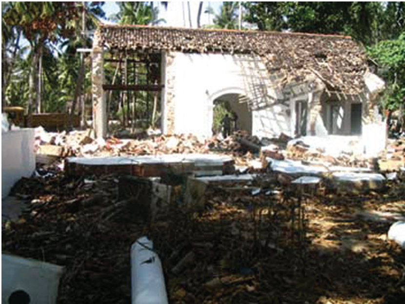
Figure 2.7 Damage caused by the 26 December 2004 tsunami at Unawatuna, Sri Lanka where the inundation depth was about 5 m. Damage to a masonry building. Source: EEFIT. Reproduced with permission.
