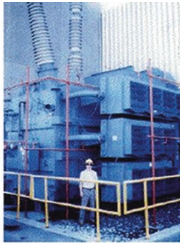
PJM Public Service Step Up Transformer
