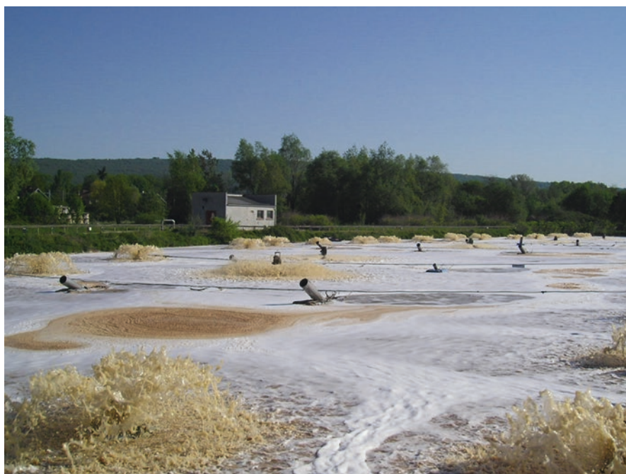
Figure. An aerated lagoon to treat wastewaters from a pulp and paper industry; source: G. Crini
