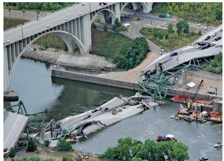
1.2 Collapsed Saint Anthony Falls Bridge in Minneapolis (USA, 2007) due to incorrectly designed joints (gusset plates) in the truss.
