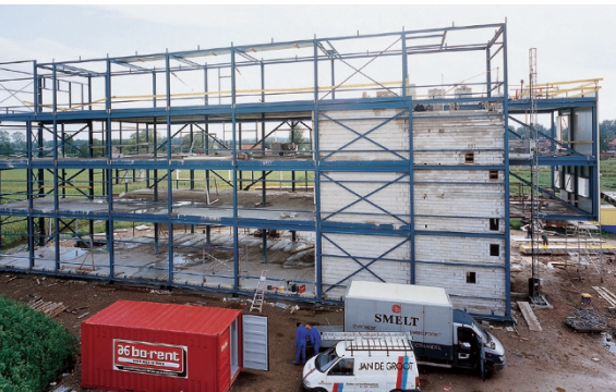
1.6 Example of permanent load: self-weight of the structure (columns, beams, floors and walls).
