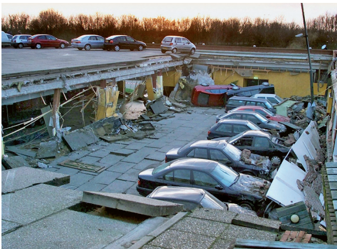
1.1 Collapsed parking deck at a hotel in Tiel (The Netherlands, 2002) due to, amongst other things, insufficient stability of the edge beam.
