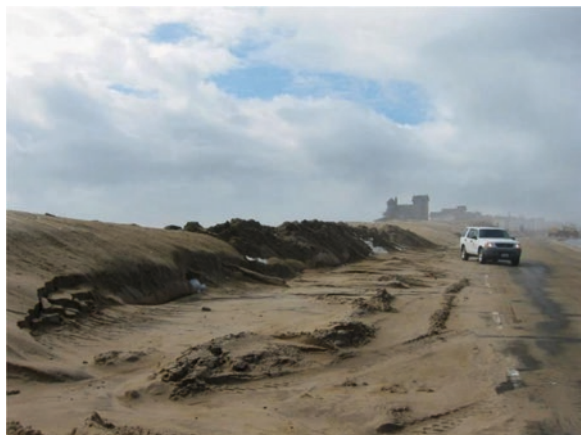
Fig. 1.10 Highway 12 just north of Rodanthe, North Carolina, looking south, showing the artificial dune on the left that was overwashed by water and sand during a nor'easter. Note the location of the white dashed line down the middle of the road. In the right distance, bulldozers are clearing sand off the highway. (Image by S.J. Culver)
