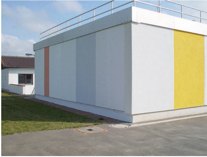
Fig. 2.3 View of the whole wall construction with attached ETICS facing west (Hofbauer et al. 2006; Hofbauer 2007)
