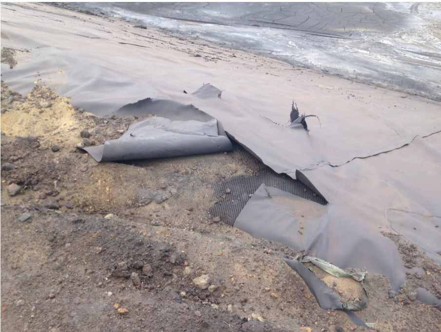
Fig. 1. A typical liner failure (Courtesy of Iluka Resources, WA, Australia).
