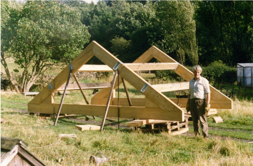
Paul working on barn roof, 1994 and the finished barn. He started building it in 1988 towards the end of the Cold War. He thought it would take three years but it took him ten, by which time a new global disorder had emerged. Source From the author’s personal photo collection
