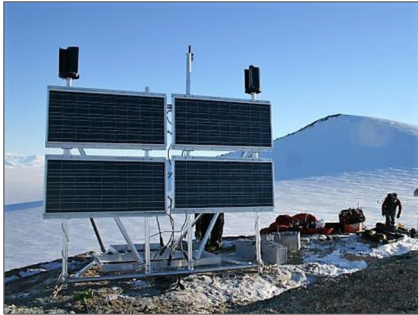
Figure 2.2 PV anywhere on earth – even Antarctica [21] where the modules are vertical.
